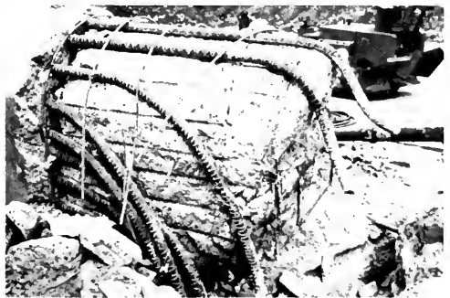
Photo 15. Failure at base of column supported on spread footing, Golden State Freeway and Foothill Freeway interchange [4].
